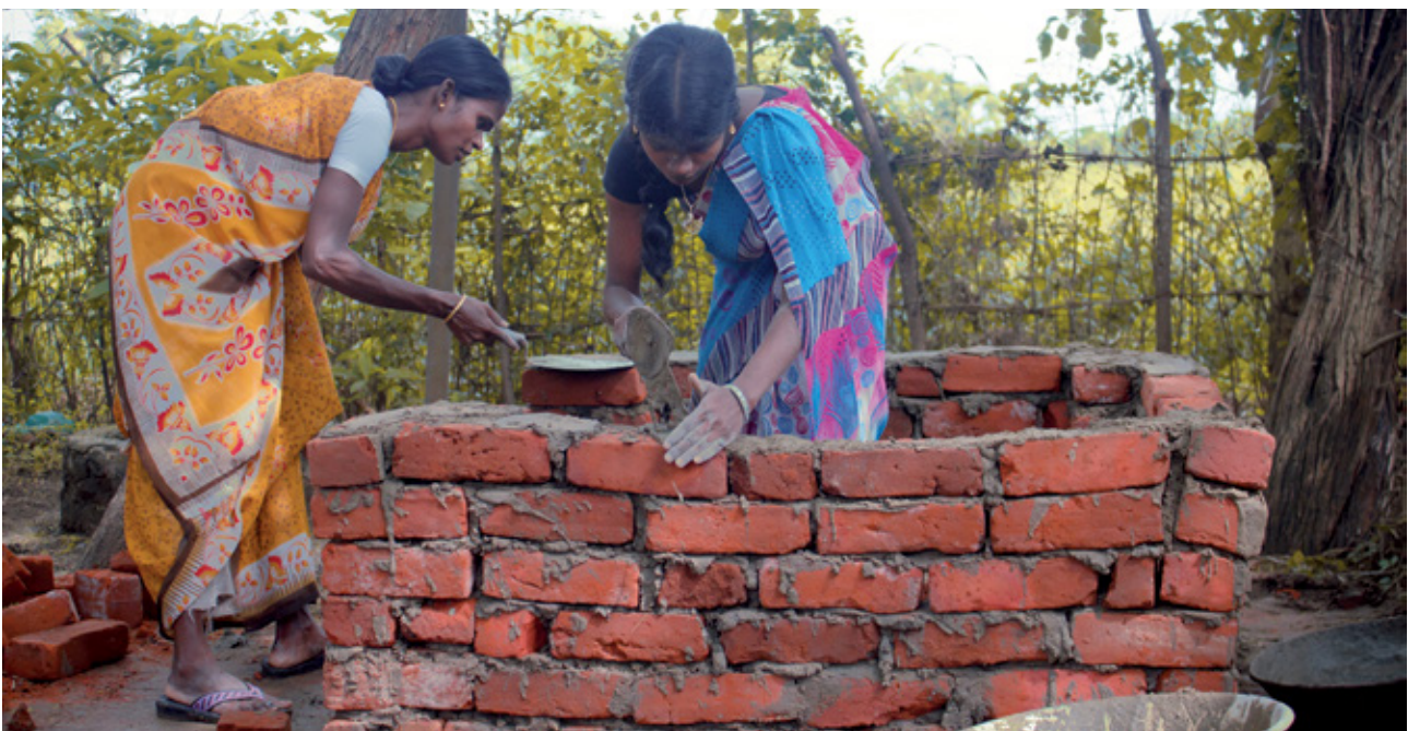
Mrs Maithili and Miss Pechiyamml working on the construction of a toilet in Kachanam village
